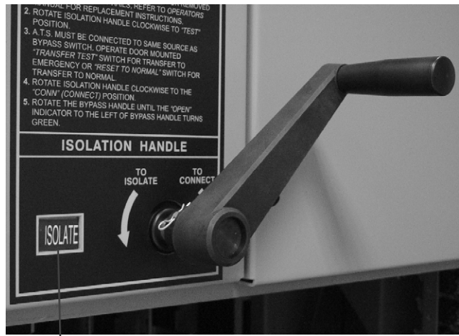
position window CONN TEST ISOLATE counterclockwise – draws out the transfer switch
