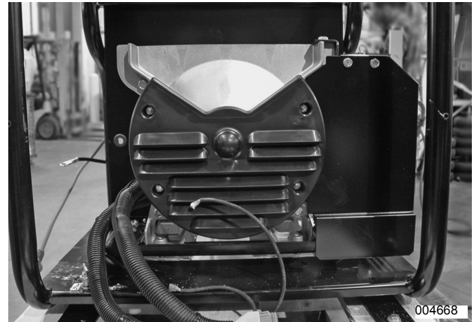
Figure 5-3. Control Panel Removed
