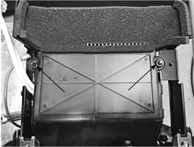
Figure 1-73. Inverter Inlet Duct
