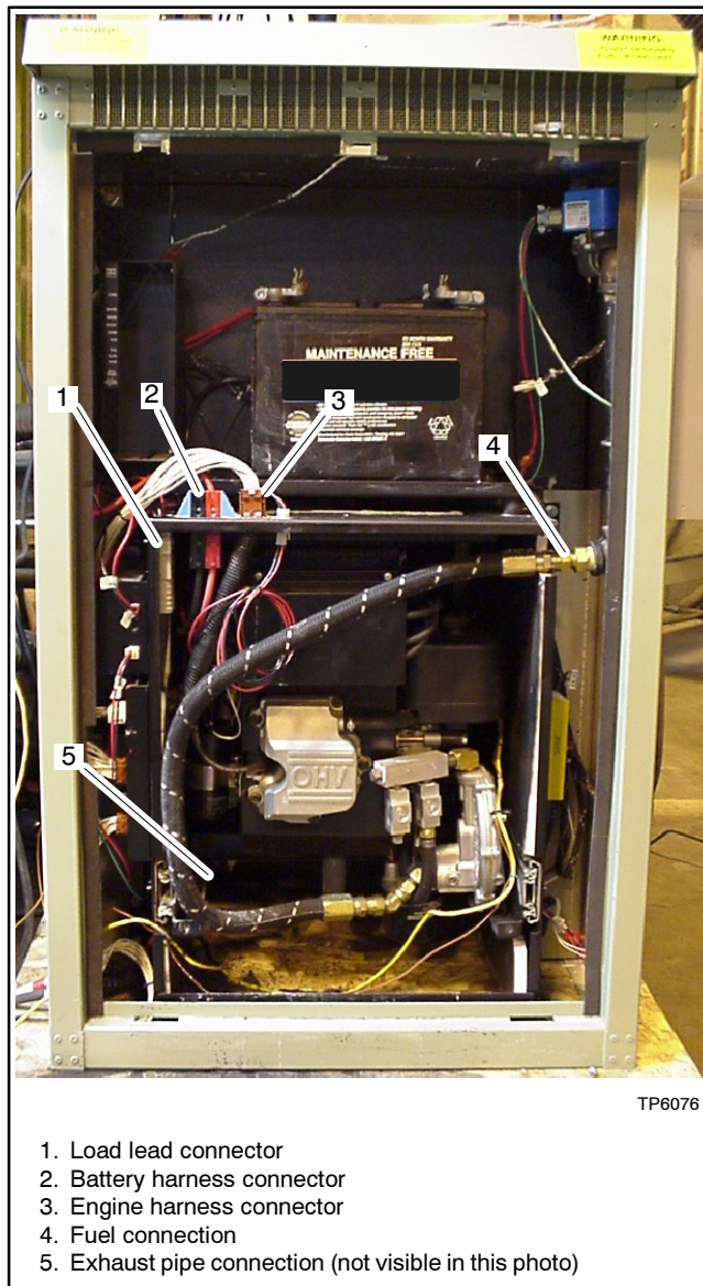
Figure 3-2 Generator Set Installed in the Cabinet
