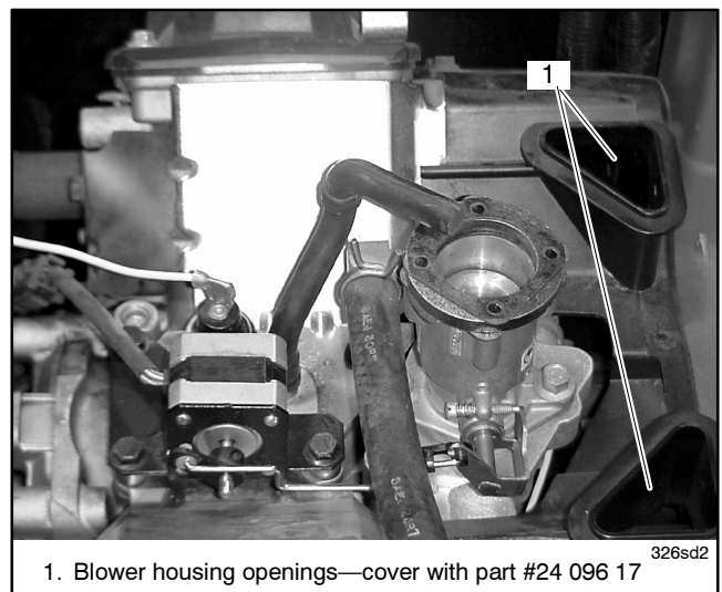
Figure 6 Blower Housing Openings
