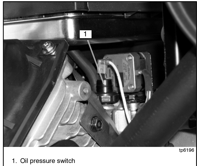
Figure 5-18 Oil Pressure Switch Location (under the air cleaner)
