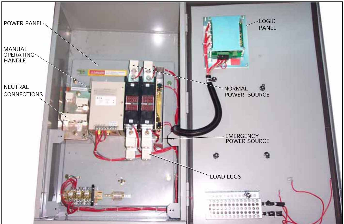
Figure 16. 400 A, 2-Pole, ATS Interior Components.
