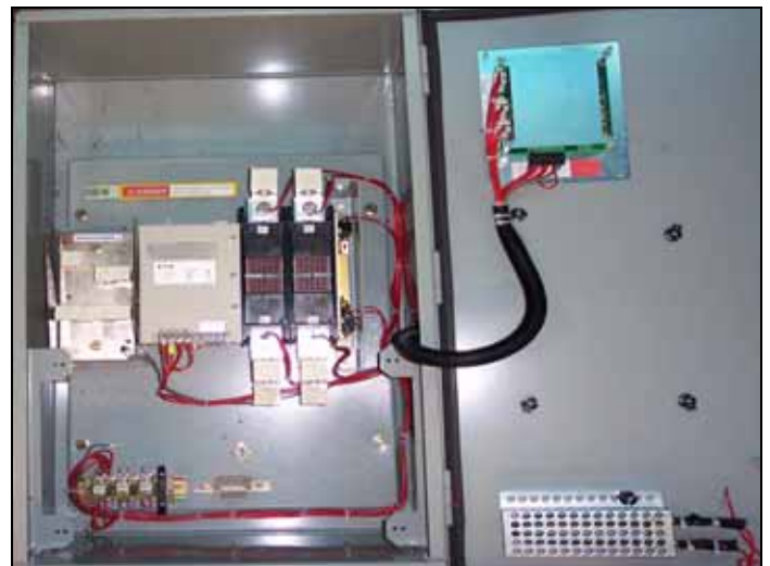
Figure 3. Typical 400 A ATS.
