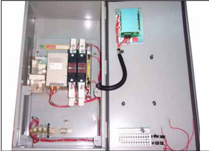
Figure 5. Typical Power Panel for 400 A Model.
