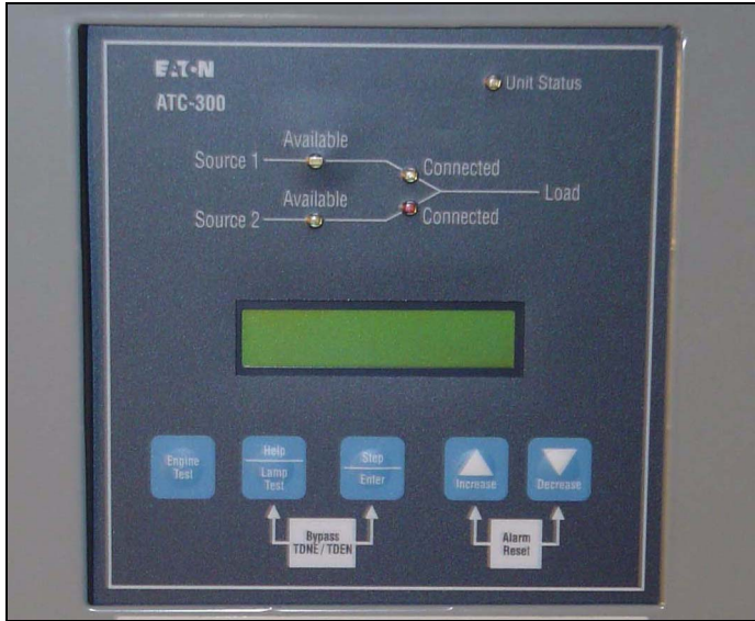
Figure 1. The ATC-300 Controller Front Panel.
