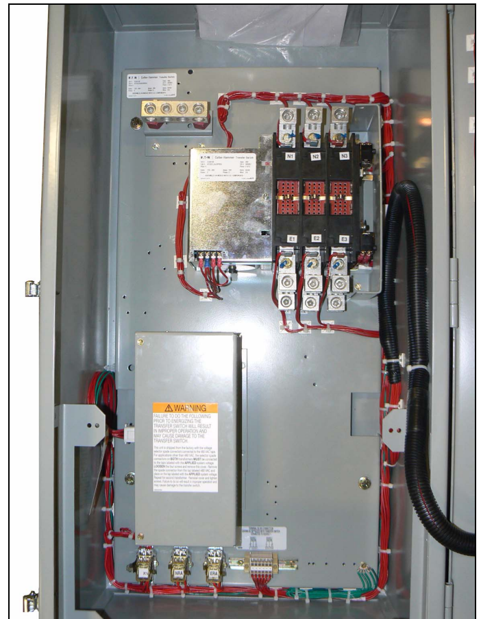
Figure 3. Typical Power Panel for a 100A Model.
