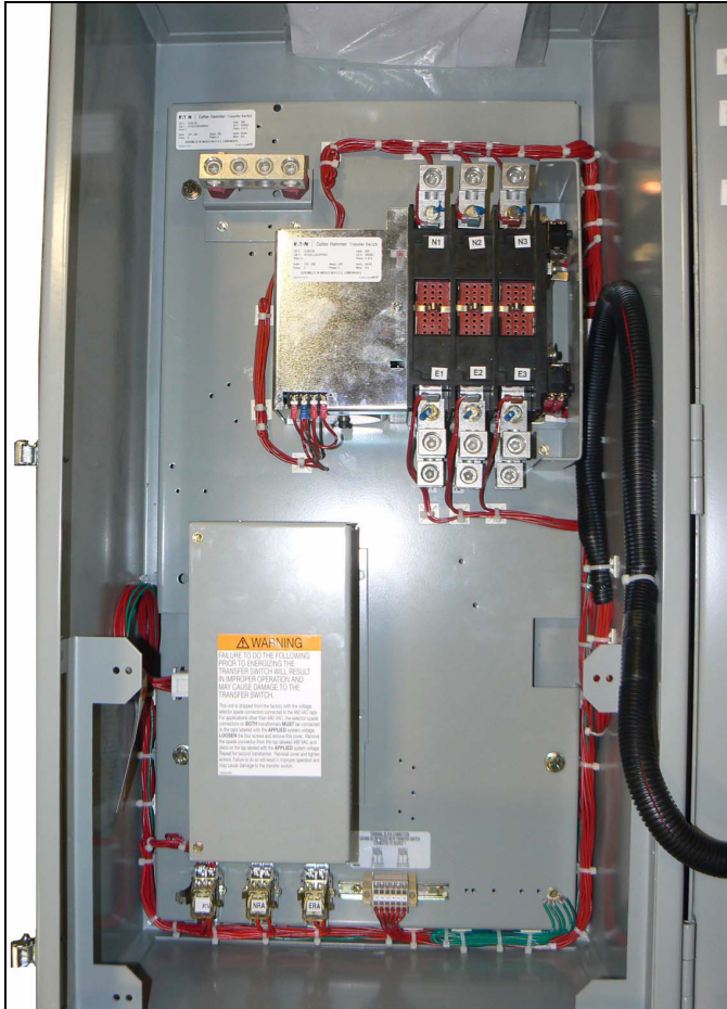
Figure 4. Contactor Based ATS (100A).
