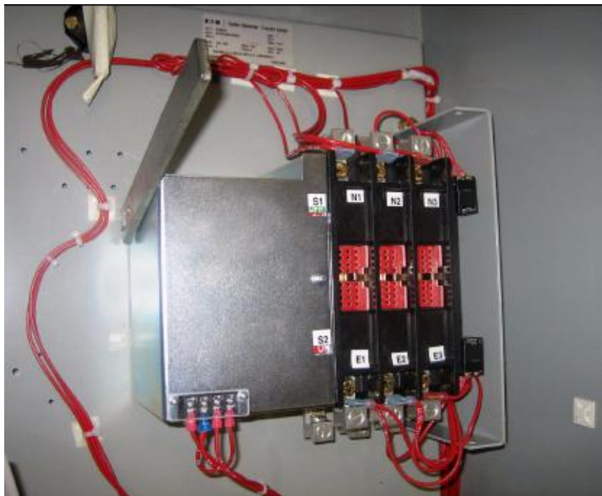
40-400 Amp Manual Operator Handle Installed
