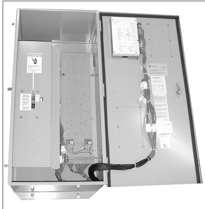
Figure 1-2 Automatic Transfer Switch Equipment with Solid Steel Shield in Place over Power Panel
