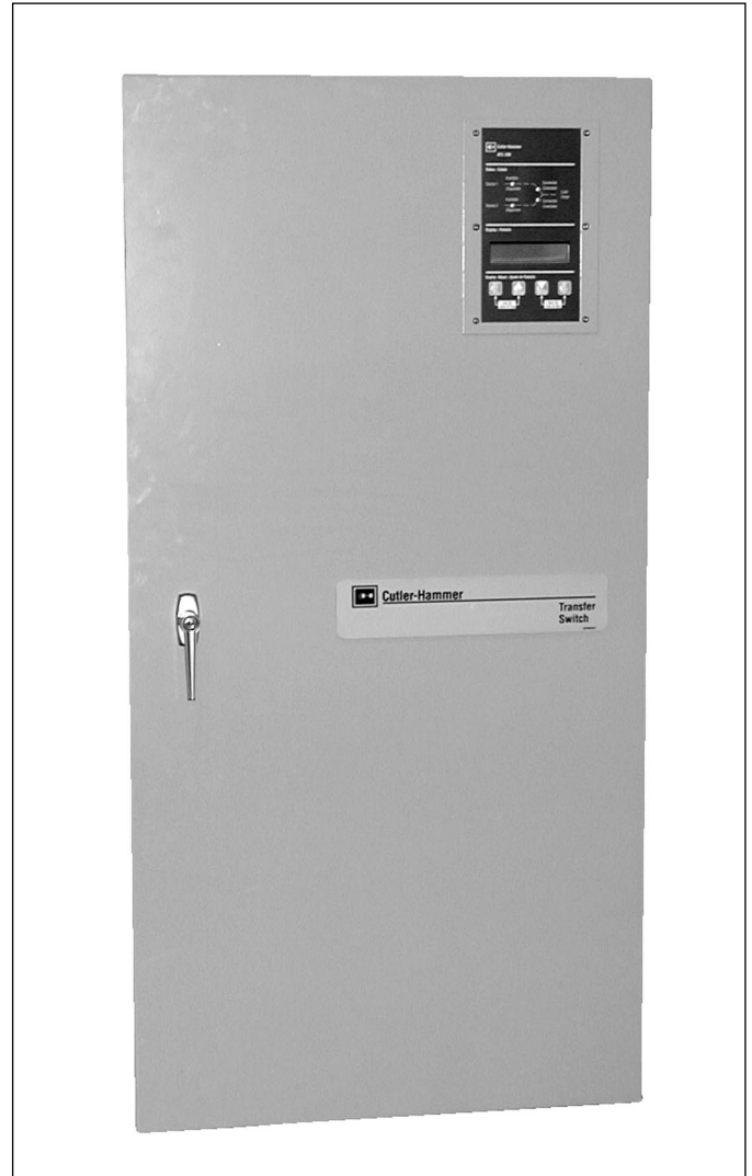
Figure 3-5 Typical Type 3R Enclosure (Door)
