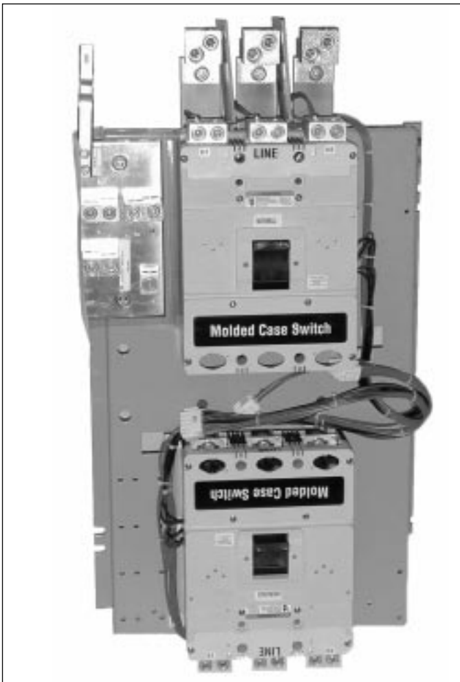
Figure 3-3 Mounted Molded Case Switches with the Transfer Mechanism Removed for Clarity (300-600A Models)
