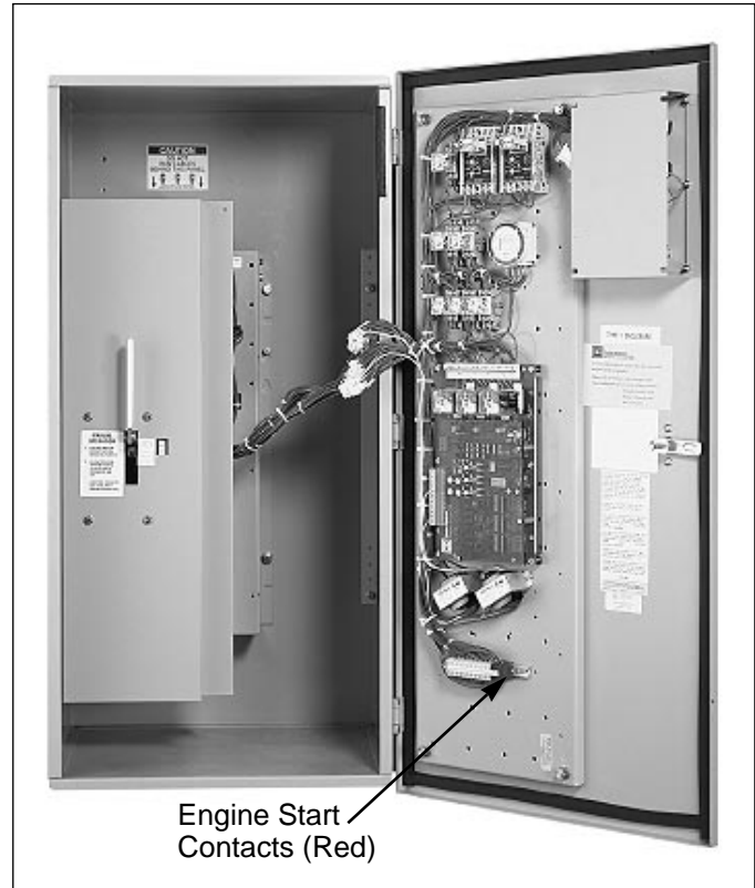
Figure 1-2 Automatic Transfer Switch Equipment with Solid Steel Shield in Place over Power Panel
