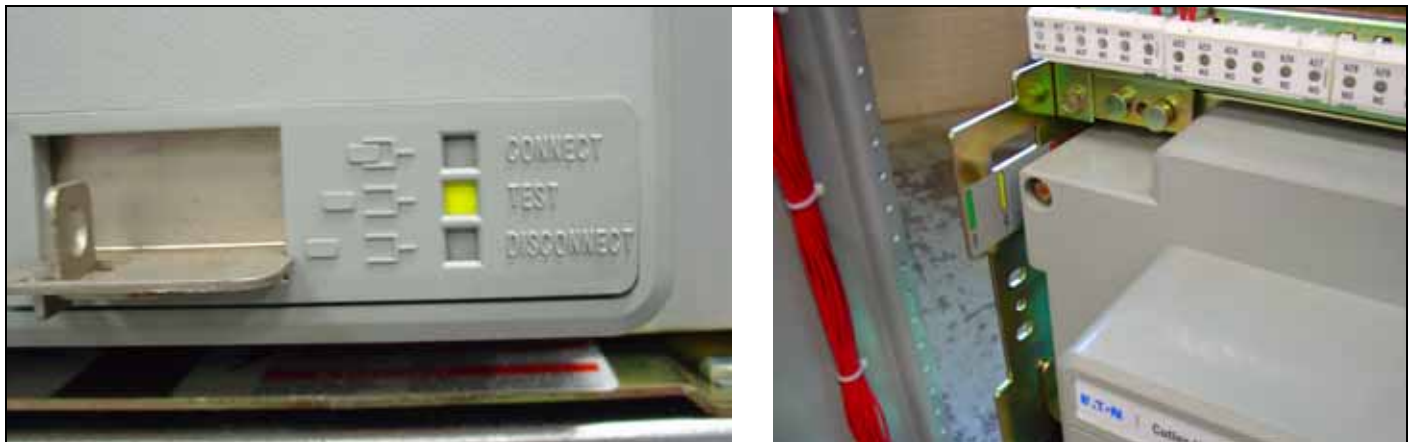
Figure 30. Switching Device in the TEST Position.
