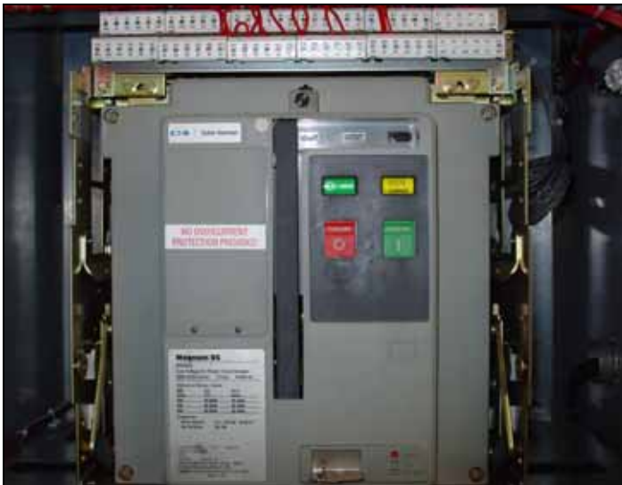
Figure 8. Drawout Switching Device Installed in the Magnum Transfer Switch.
