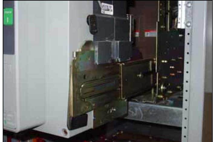
Figure 28. Switching Device in the REMOVE Position.
