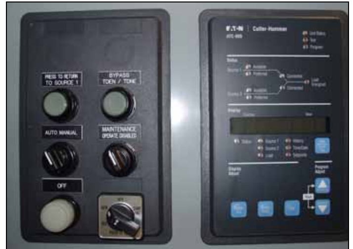
Figure 35. Bypass Isolation Switch.
