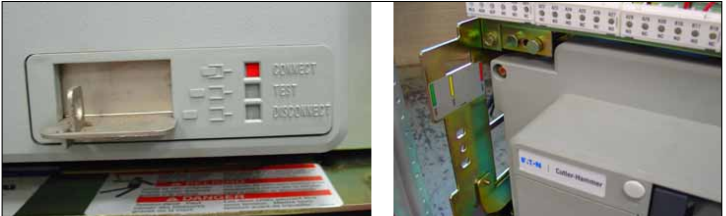
Figure 29. Switching Device in the CONNECT Position.
