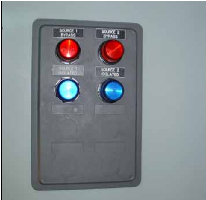
Figure 36. Magnum Bypass Lights.
