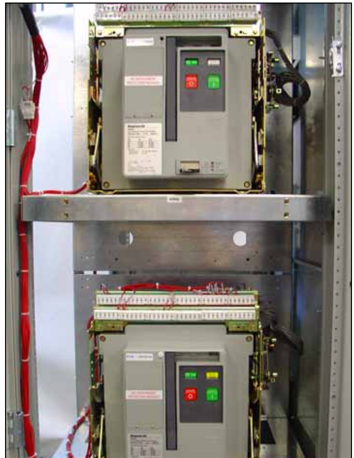
Figure 11. Typical Power Panel (Open Transition Shown).
