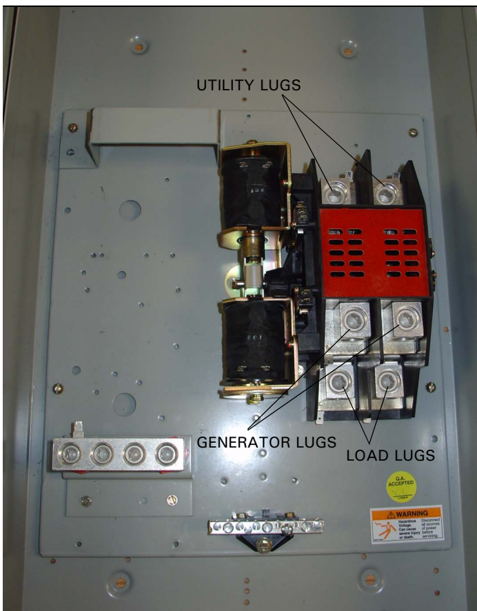
Figure 13. Cable Connection Locations (200 A).
