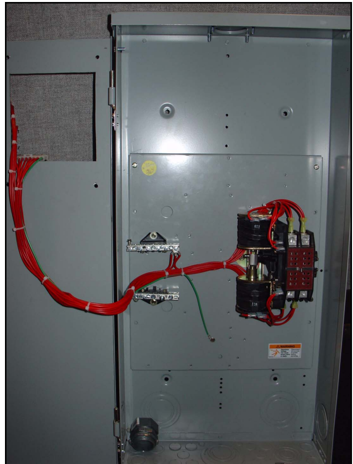
Figure 6. Typical Power Panel for 100 A Model.
