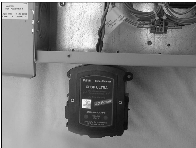
Figure 9. TVSS Mounted to the Outside of a Standard Enclosure.
