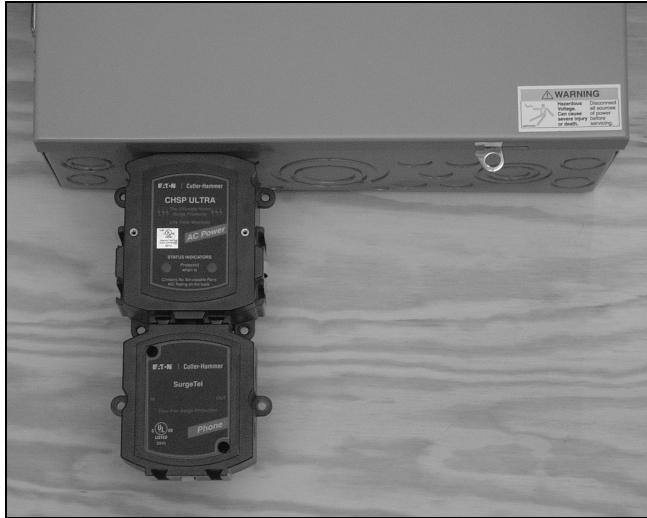
Figure 61. SurgeTel Installed with the ATS and TVSS System.
