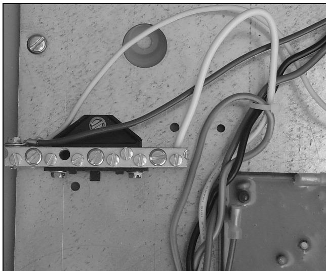
Figure 95. Load Shed Wire Connected to the Neutral Bar (100 A).
