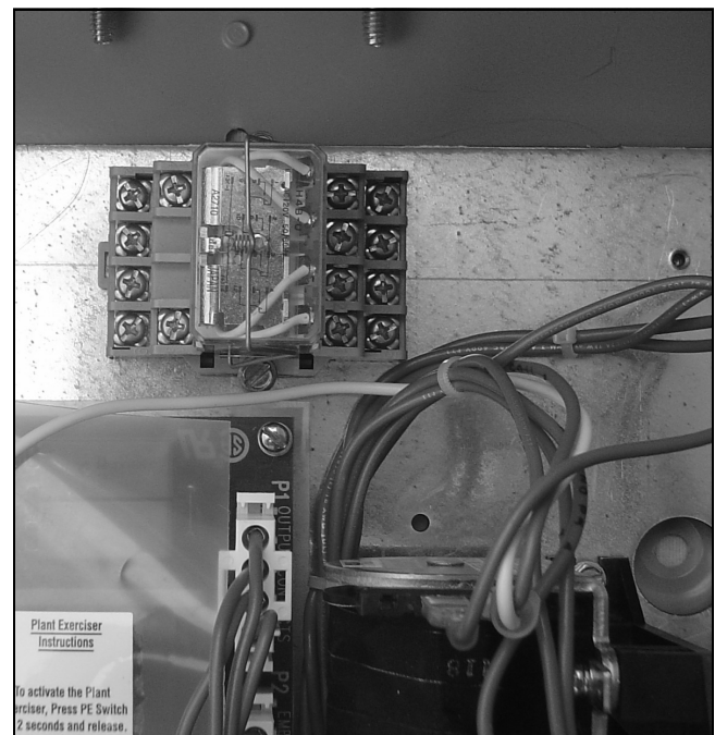
Figure 93. Load Shed Installed in a Standard ATS.
