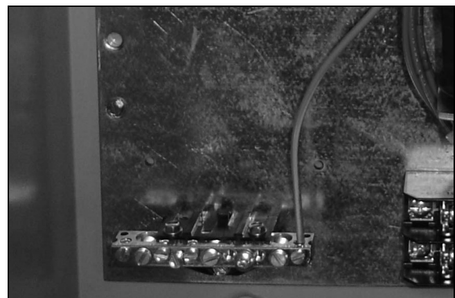
Figure 87. TVSS Green / Yellow Wire Connected to the Ground Bar.
