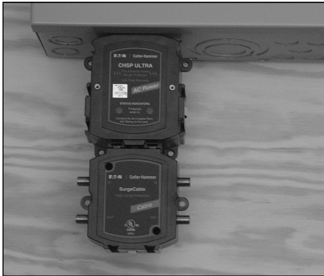
Figure 91. SurgeCable Installed on the TVSS.
