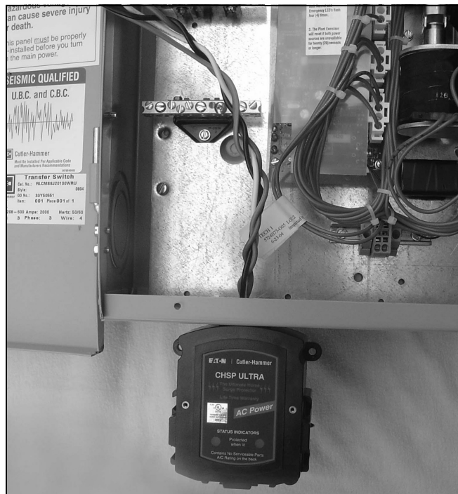
Figure 72. Possible Location for and Externally Mounted TVSS.
