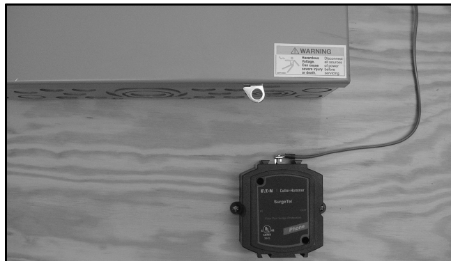
Figure 62. SurgeTel Installed Separate from the TVSS.
