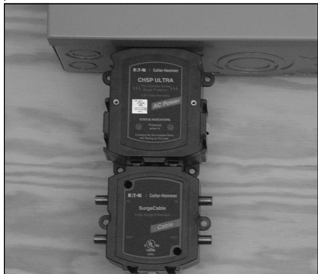
Figure 64. SurgeCable Installed with the ATS and TVSS System.
