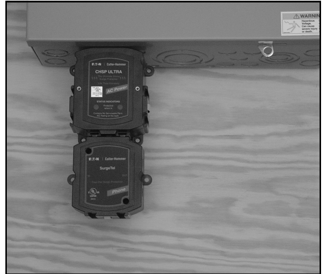
Figure 89. SurgeTel Installed on the TVSS.
