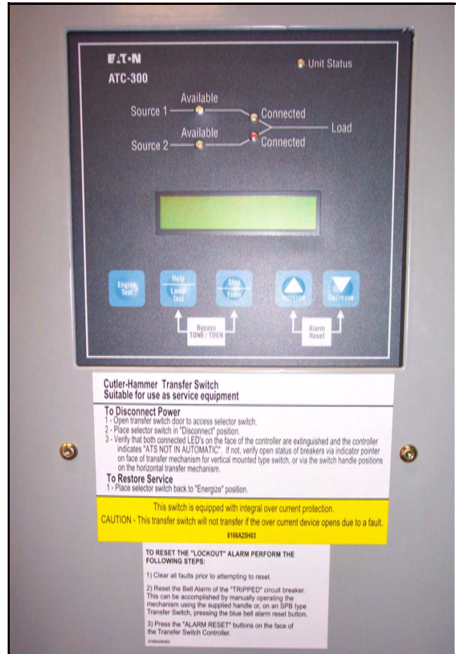
Figure 15. ATC-300 Logic Control Panel.
