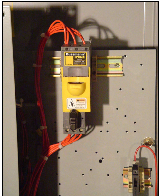
Figure 47. Source 1 Control Disconnect in the ON Position.
