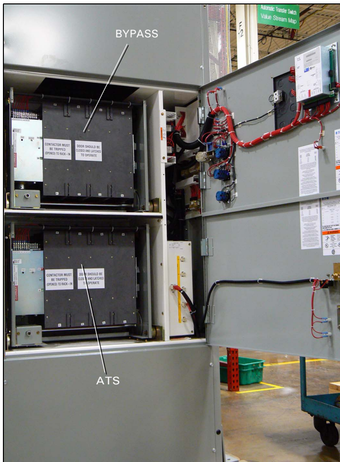
Figure 5. Switching Devices Installed in the Transfer Switch.
