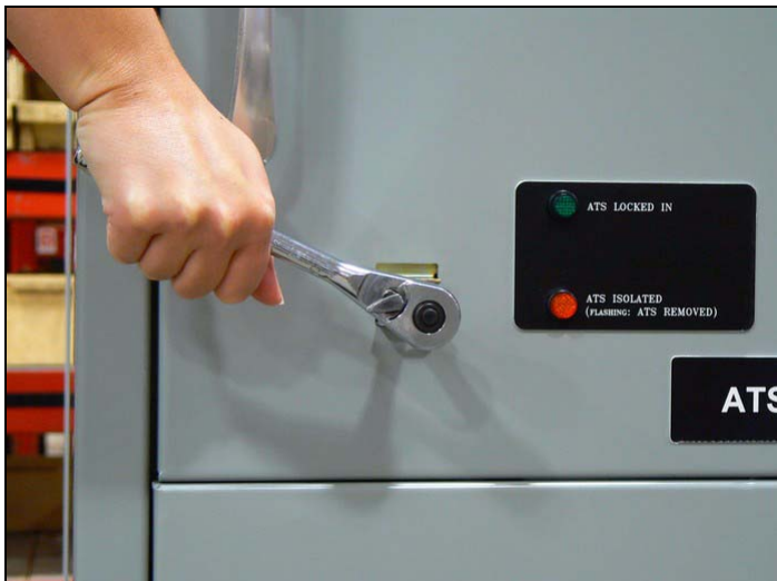
Figure 33. Levering the Contactor into its Different Positions Using a Clockwise Ratcheting Motion.
