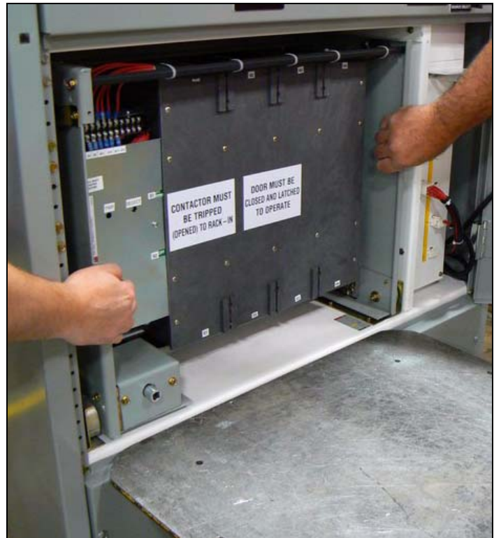
Figure 6. Draw-out Switching Device Fully Extended from the Transfer Switch's Runbacks.
