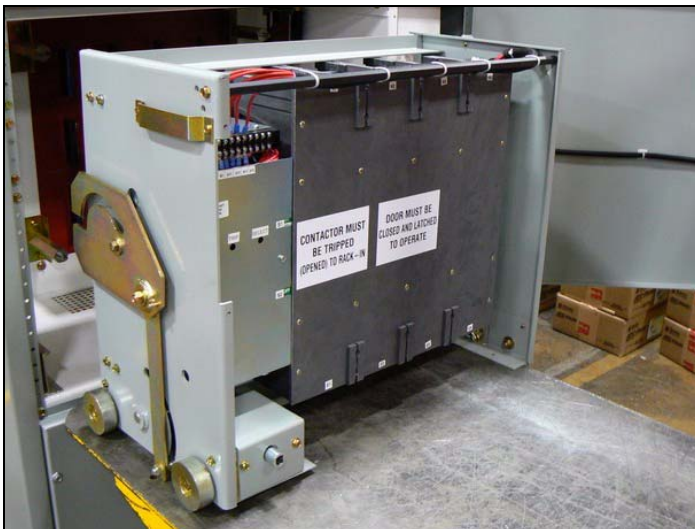
Figure 36. Contactor Rolled Out from the Rails of the Cell.
