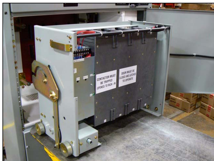
Figure 44. Contactor Rolled-out from the Rails of the Cell.
