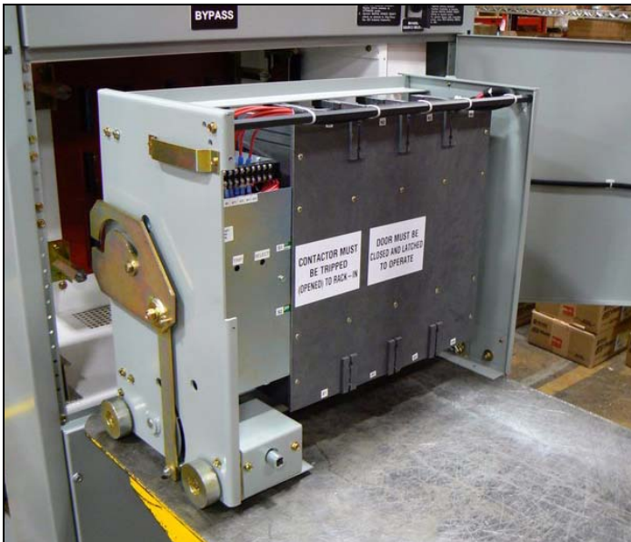
Figure 30. ATS Contactor Device Drawn-out from the Transfer Switch.
