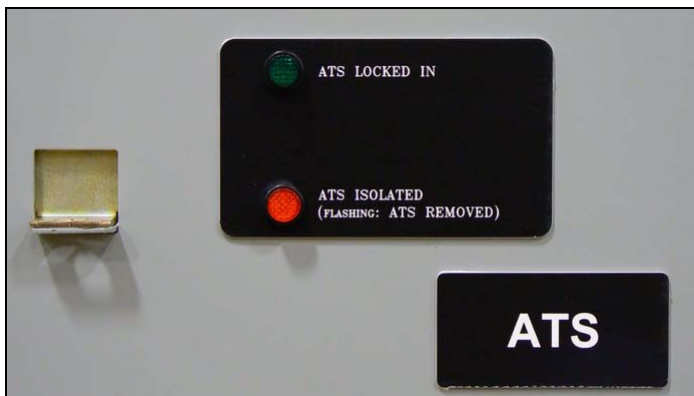
Figure 26. Bypass Bottom Lights.
