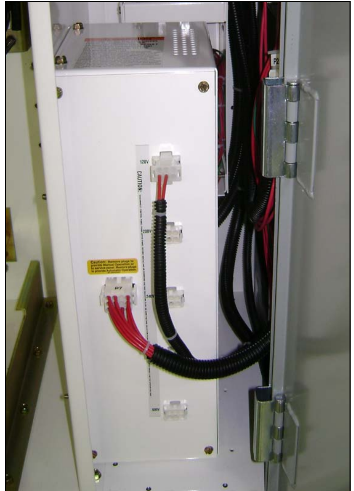
Figure 14. Transformer Selection Terminals (Shown Connected to the 120 Vac Tap).
