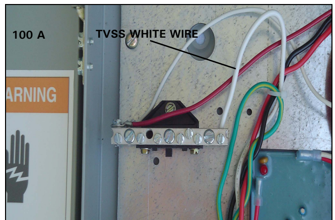
Figure 68. TVSS White Wire Connected to the 100 A Neutral Bar.
