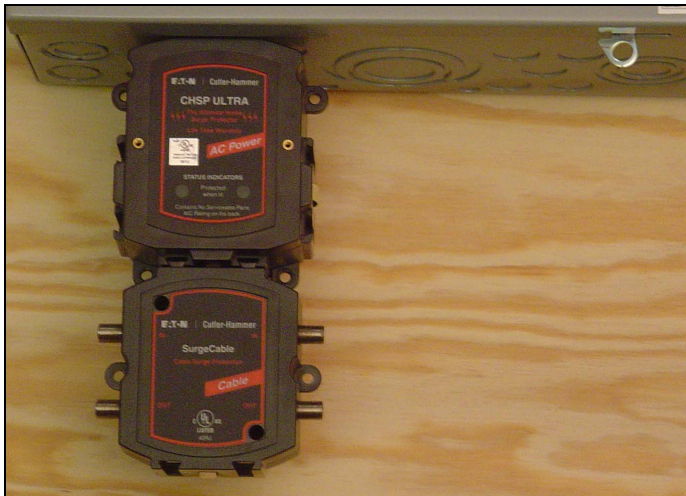
Figure 77. SurgeCable Installed on the Externally Mounted TVSS.
