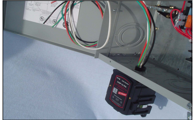
Figure 54. TVSS Secured to the ATS Enclosure.
