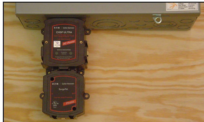
Figure 72. SurgeTel Installed on the Externally Mounted TVSS.
