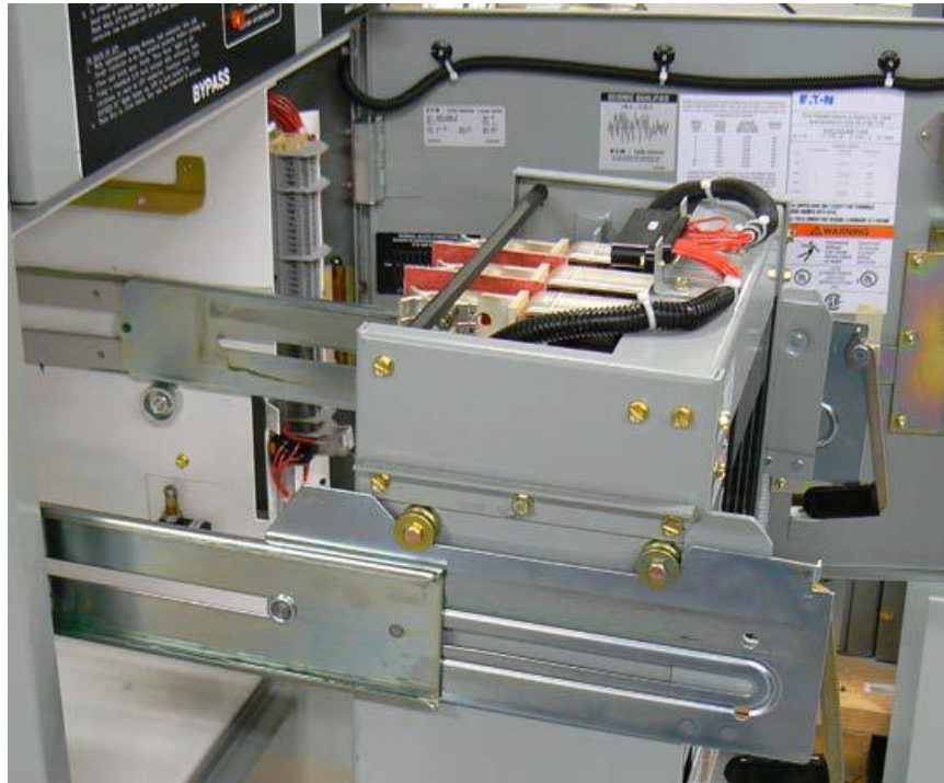
ATS Drawout Contactor in the Drawn Out Position
