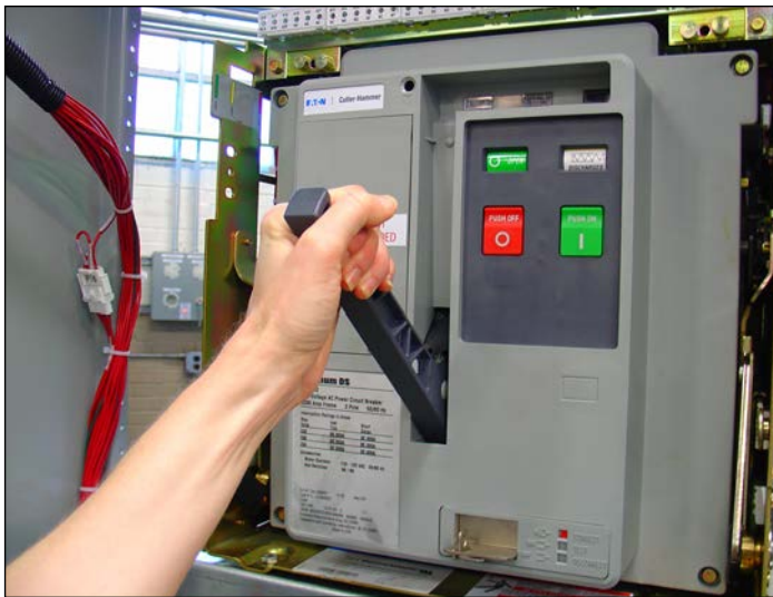
Figure 24. Pumping Handle Charges Stored Energy Mechanism (Closed Transition Shown).
