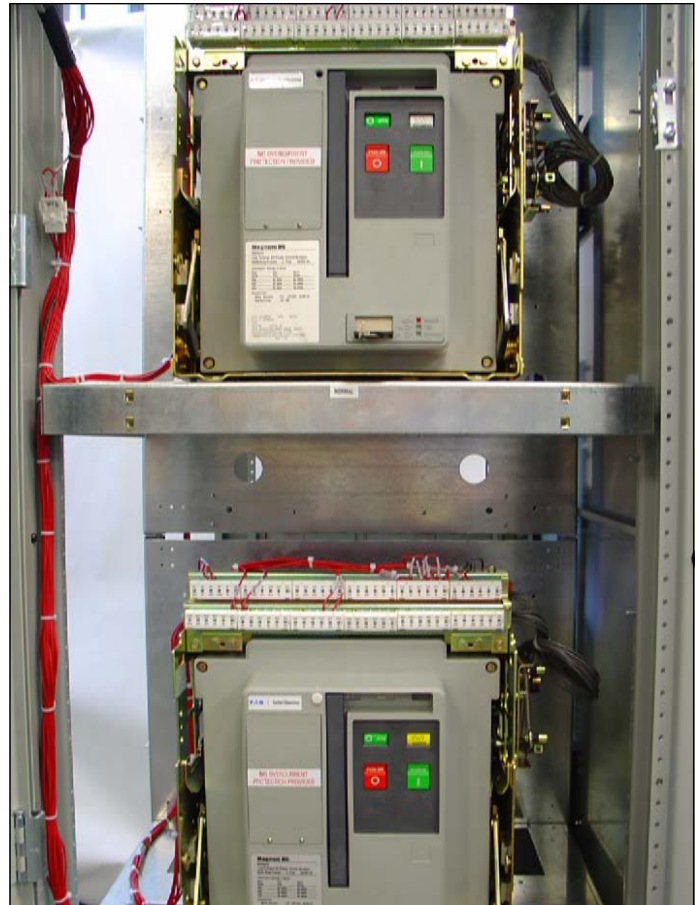
Figure 11. Typical Power Compartments (Open Transition Shown).
