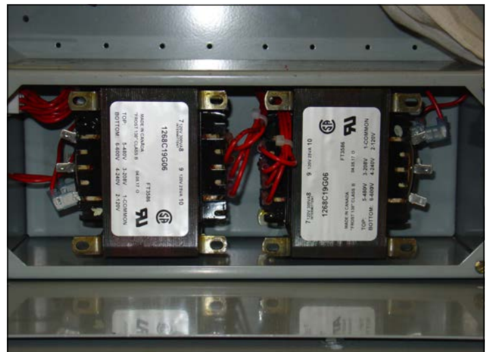
Figure 16. Power Transformers (Source1 & Source 2).
