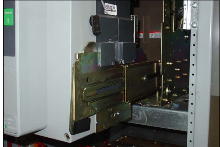
Figure 29. Switching Device in the REMOVE Position.
