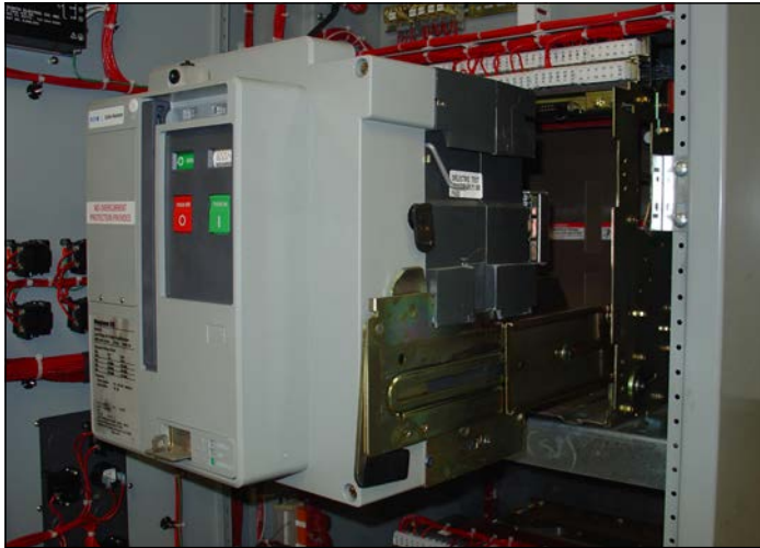
Figure 27. Switching Device Drawn Out from the Transfer Switch.
