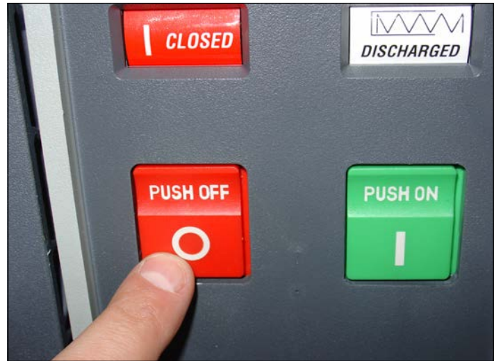
Figure 25. Close Switch by Pushing Close Button.
