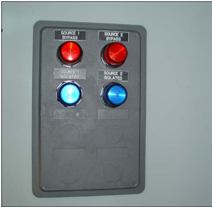
Figure 37. Magnum Bypass Lights.
