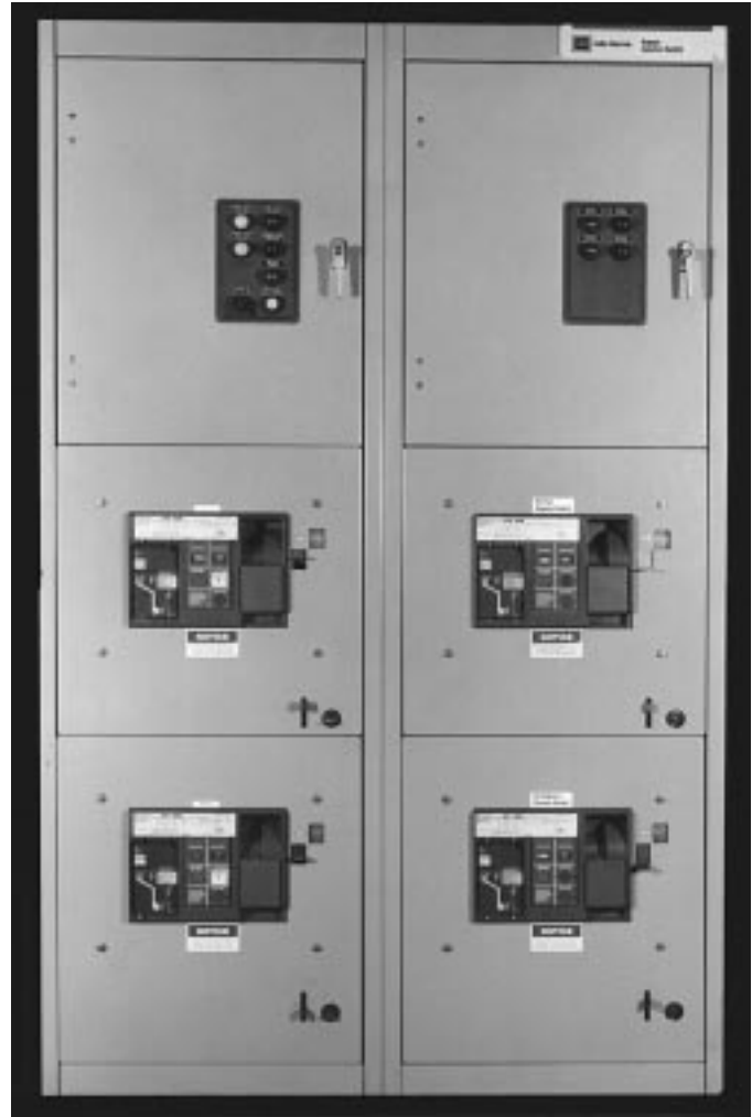
Figure 7-1 Bypass Isolation Switch
