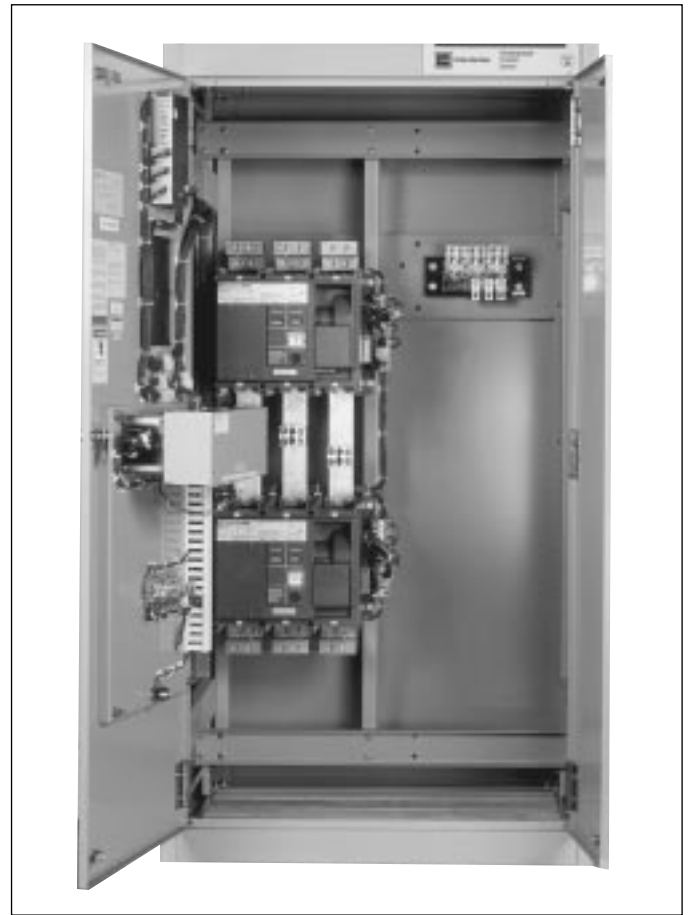
Figure 1-3 Typical Mini Transfer Switch with Dead Front Removed
