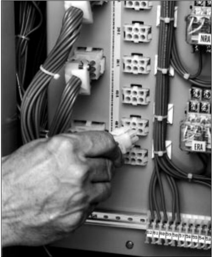
Figure 3-4 Vertical Design Voltage Selection Panel with Voltage Being Selected
