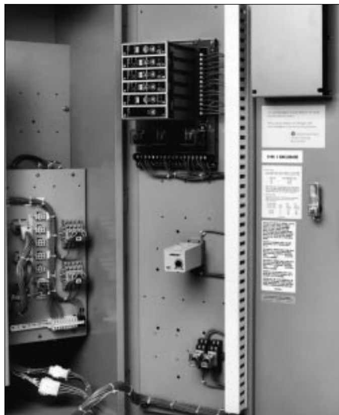
Figure 3-5 Typical Solid State Logic Panel (Door Mounted)
